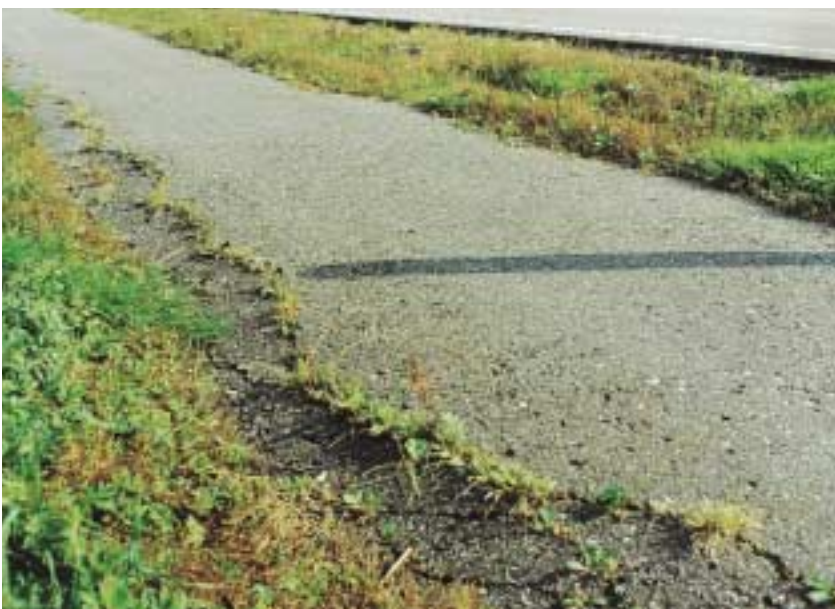
A poor construction narrows the cycle track and path.
