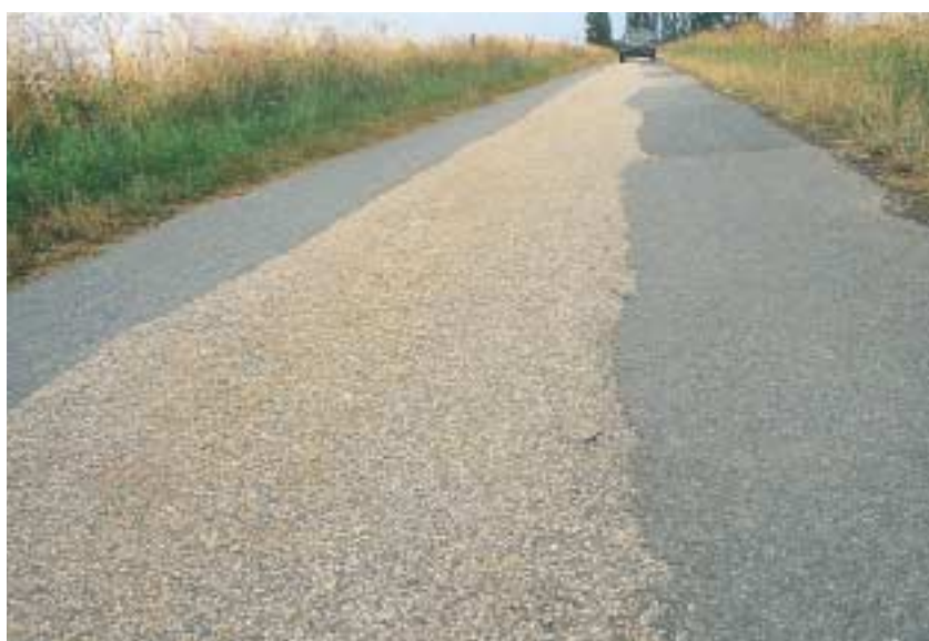
Road with many patches (repairs).
