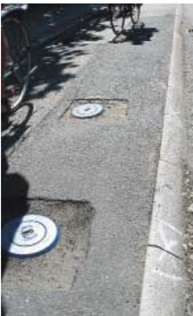
A warning about these holes is necessary.
